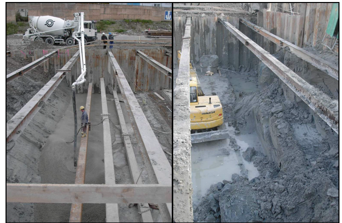
Fig. 12. Some details of construction works with slicewise excavation and placement of bottom slab
