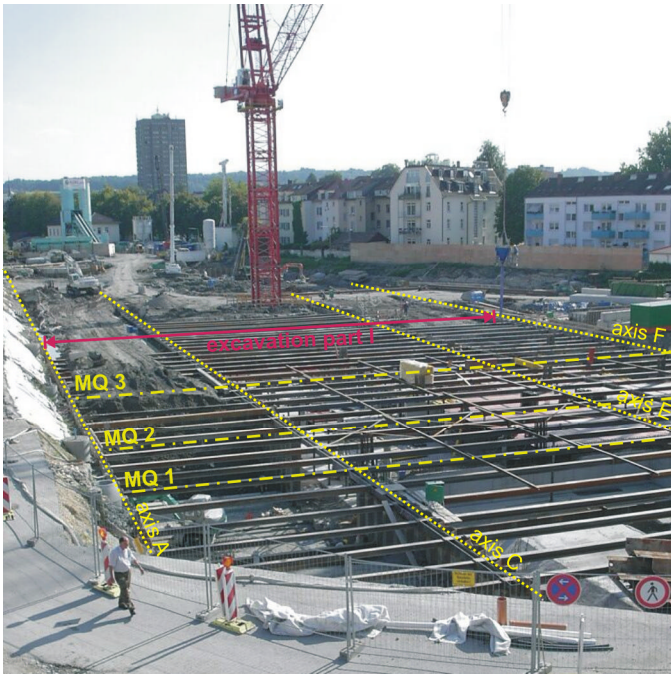
Fig. 10. Execution of the strip on Hafen street side till block 6 (axis E-F)
